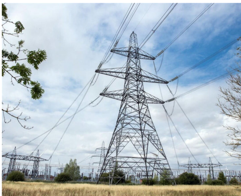
Image 5.13 Typical terminal lattice pylon 3
