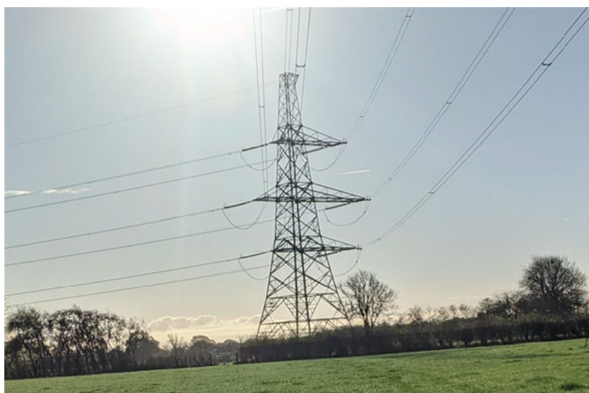
Image 5.12 Typical tension/angle lattice pylon 2
